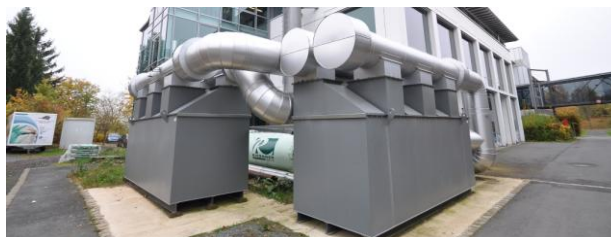
Figure 37: Storage modules of the combined TES and ORC facility at the University of Bayreuth
