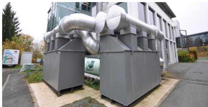
Figure 1: Storage modules of the combined TESS and ORC facility at the University of Bayreuth
