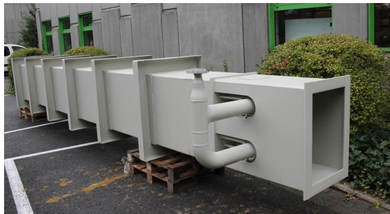
Figure 6. Picture of the LHS installed at UGhent Campus Kortrijk.
