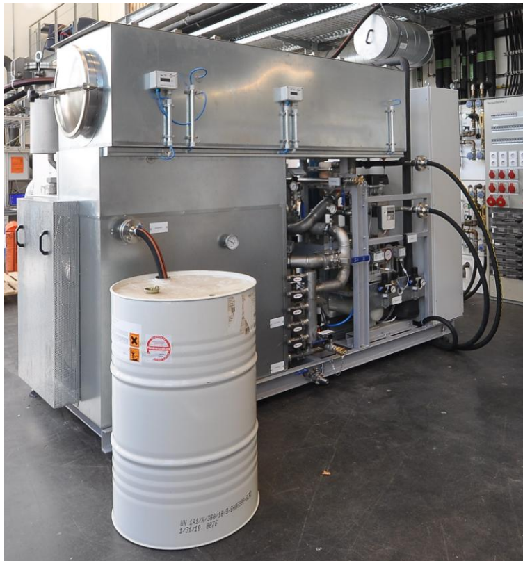
Figure 2: Demonstration unit of an HDH process for bilge water treatment
