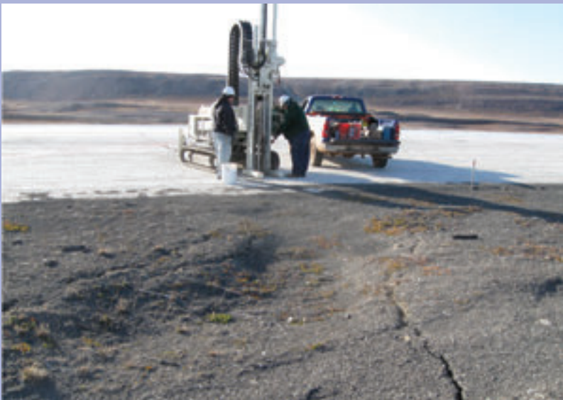
FIG. SB5.4. Thaw settlement (~0.65 m) associated with an airfield in Greenland. Thawing of ice-rich, weathered bedrock at approximately 2 m below the surface is causing severe settlement, resulting in the need for significant maintenance measures to continue operations. Photograph by Kevin Bjella.
